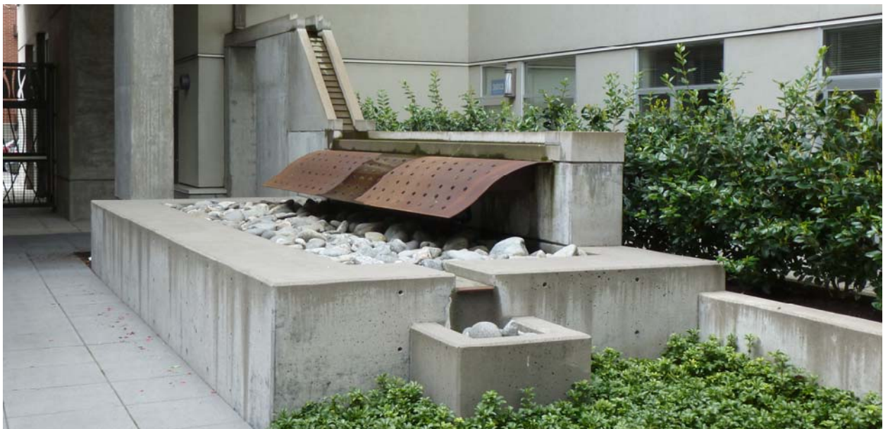
Figure 29 - Example of stormwater infrastructure incorporated into public art
